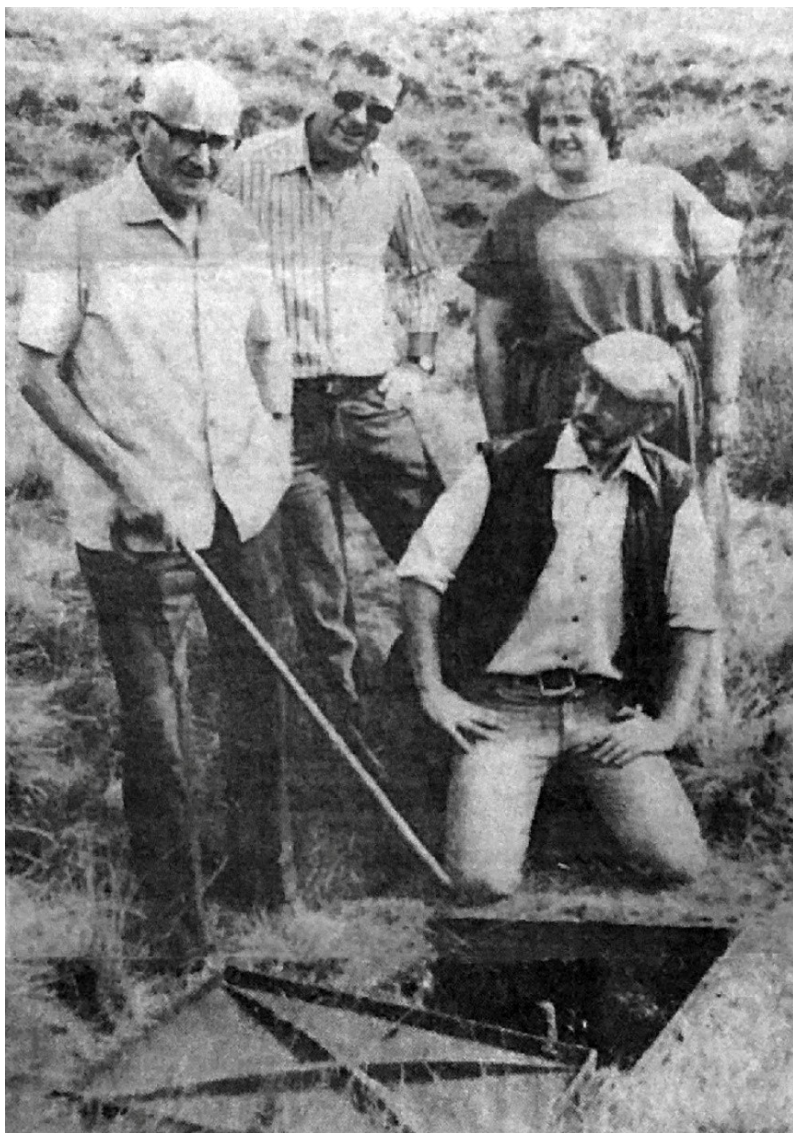
Councillor Ken Hakin (left) points out the danger of the easily lifted trap door to Councillors Doug Stanley, Kathleen Waterhouse and Mike Crompton
