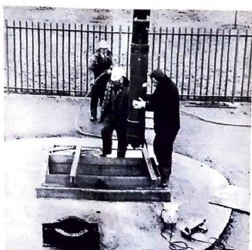
● Maintenance fitters (left to right): Sam Garratt, Ron Murden and Ron Johnson, with a little assistance from a large mobile crane, lowering a submersible motor, pump and cable into a deep well at Salford. Lengths of pipe are bolted on as the unit is lowered to join into the pumping main at Hucknall.
